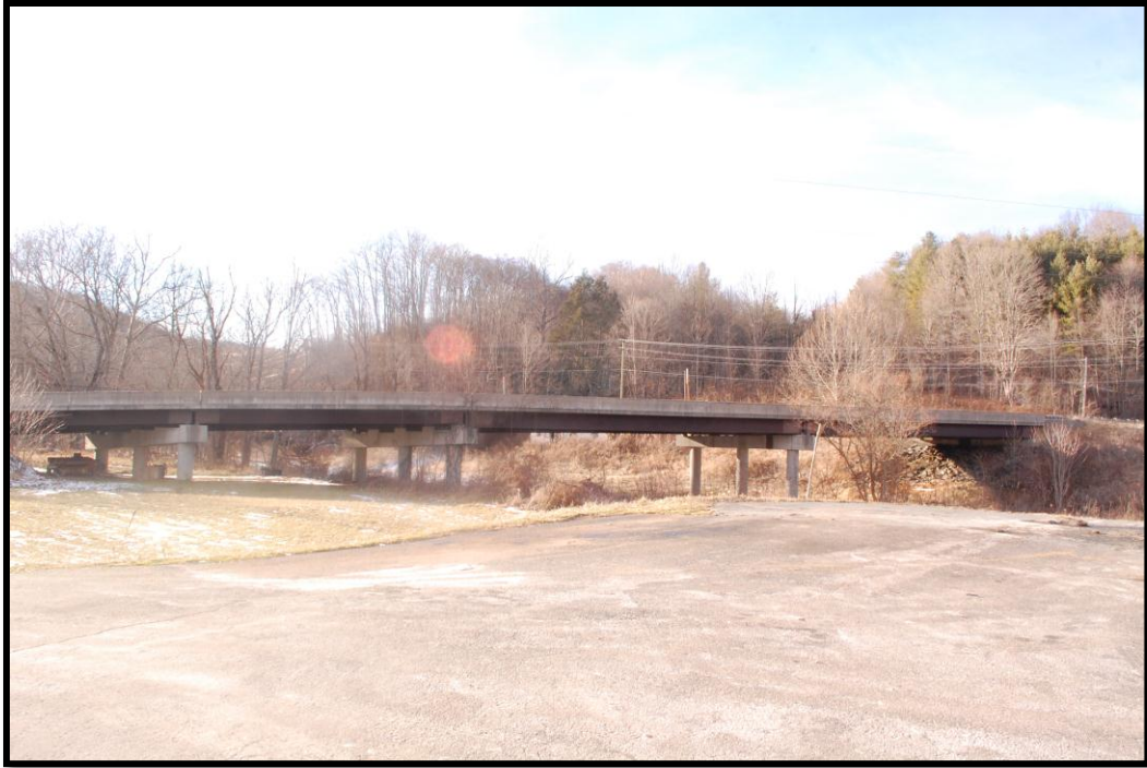
Figure 35: Bridge over North Fork of the New River, view to the west
