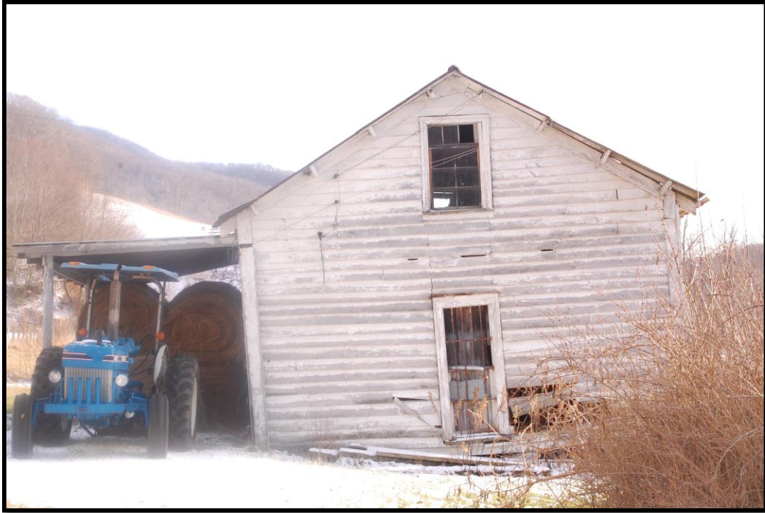
Figure 10: Equipment shed just off southwest corner of the house, view to the southeast.
