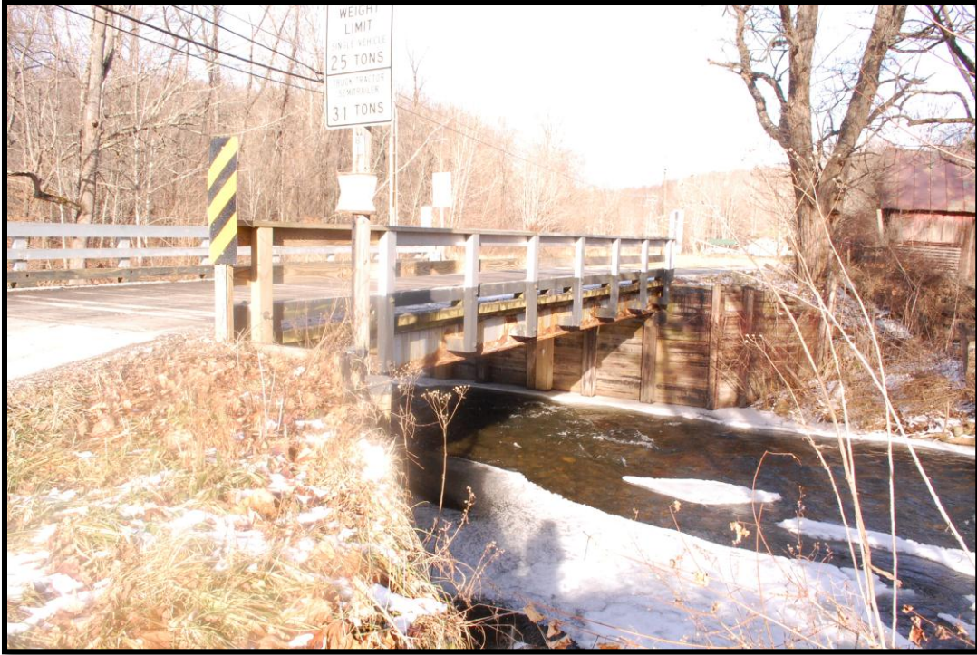
Figure 27: Bridge No. 187 and David Worth House barn (to the right), view to the east-northeast
